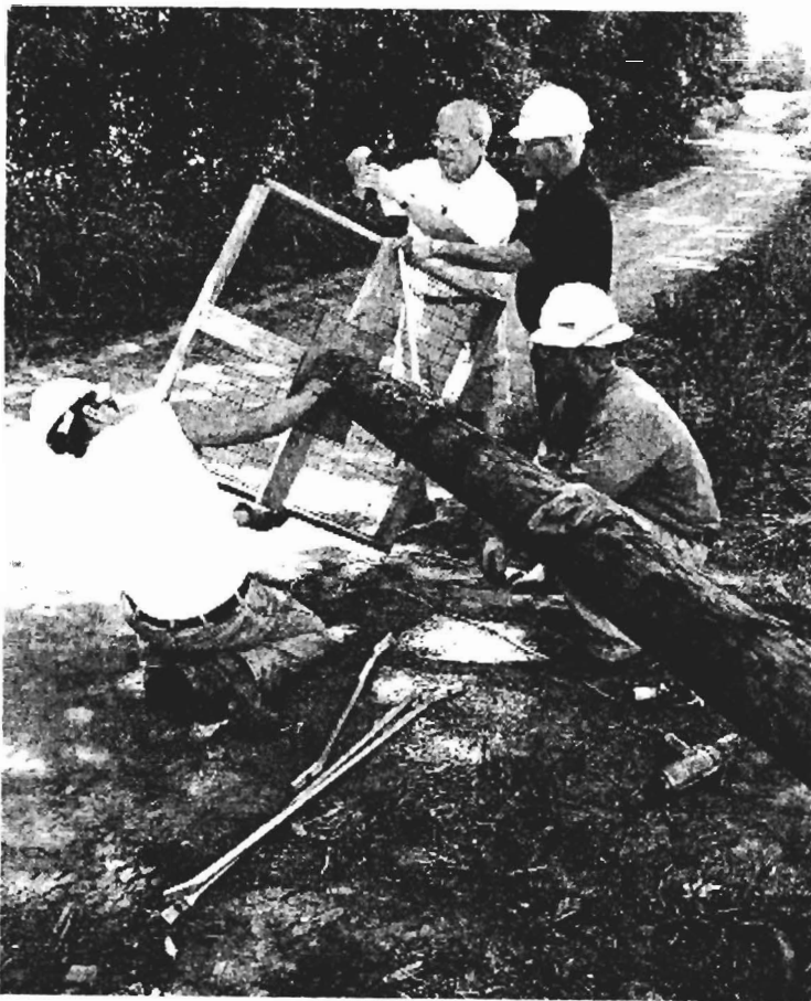
John Getzendanner, hatless, and the crew from Cinergy attach the osprey platform to the top of a 35-foot pole.
